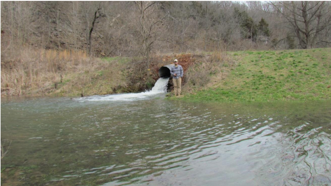
Figure 4. Discharge of 11.57 mgd from the outflow pipe at Lake Spring. This flow is almost completely leakage from the planned reservoir area that would not be prevented by the dam.
