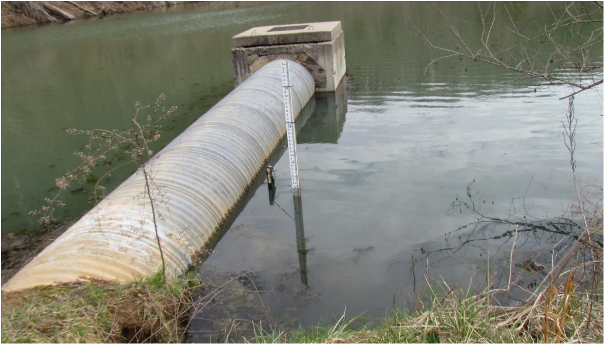
Figure 3. Flow rate measuring equipment at Lake Spring.
