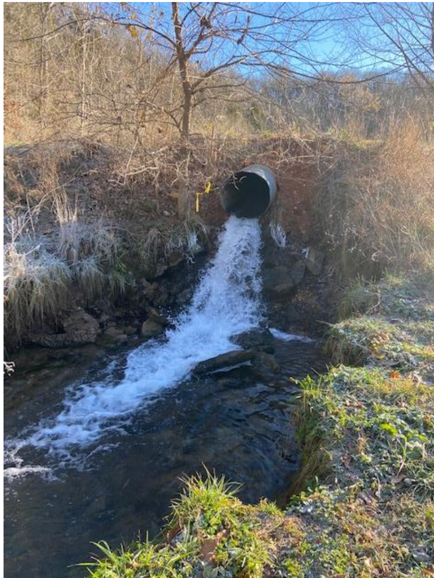
Figure 17. Hunley Lake outflow discharging approximately 2.9 mgd on December 1, 2020.
